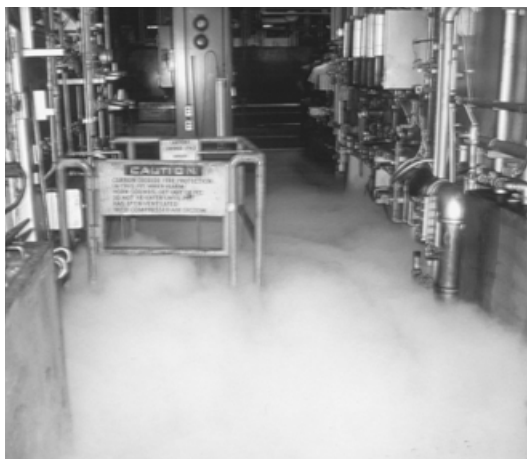
FIGURE 6.92 Carbon dioxide accumulated at floor level.
