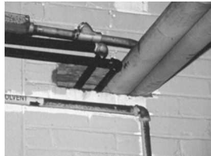
FIGURE 6.5 Unprotected opening through fire wall.
