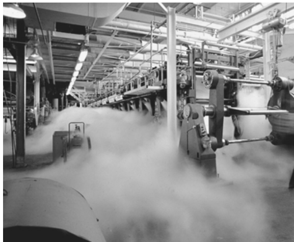
FIGURE 6.91 Carbon dioxide system discharge.
