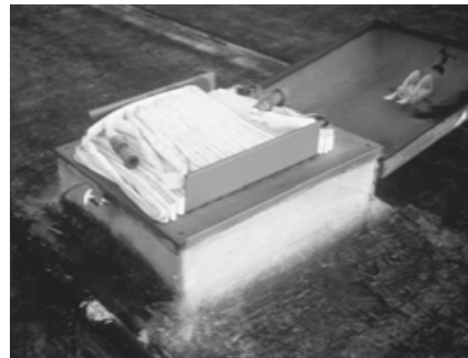
FIGURE 6.27 Roof standpipe station.
