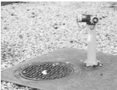
FIGURE 6.74 Fire department connection.
