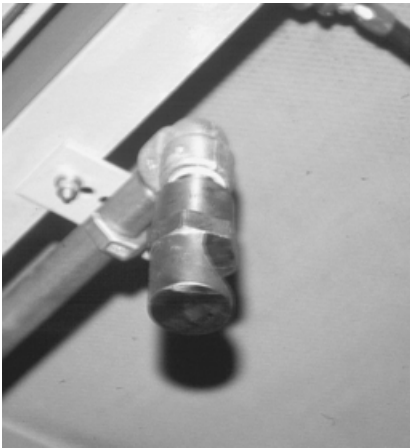
FIGURE 6.94 Halon system nozzle.
