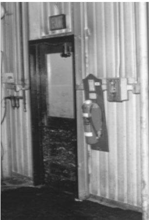
FIGURE 7.32 Extinguisher mounted near exit.
