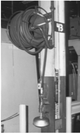
FIGURE 6.89 Carbon dioxide system hand line.
