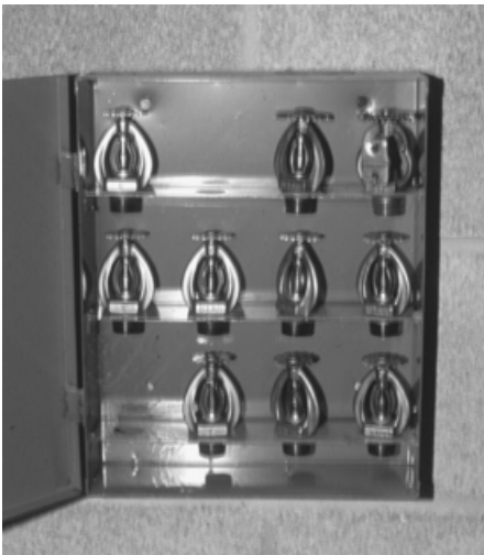
FIGURE 6.53 Extra sprinkler head cabinet.
