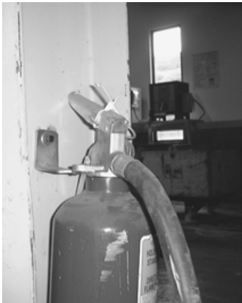
FIGURE 7.55 Extinguisher with damaged pin.
