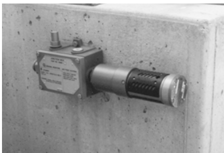
FIGURE 6.99 Flammable vapor sensor.
