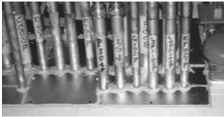
FIGURE 6.4 Fire barrier around conduit.
