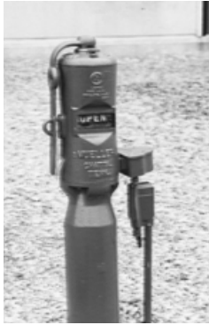
FIGURE 6.68 Post indicator valve (PIV).
