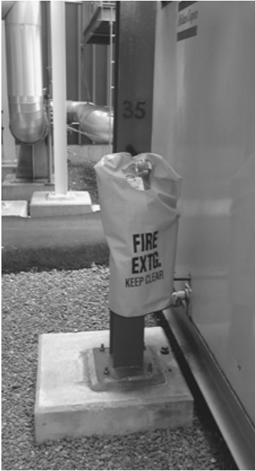
FIGURE 7.40 Extinguisher mounted outside.
