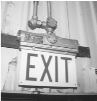
FIGURE 4.10 Exit sign for hazardous location.
