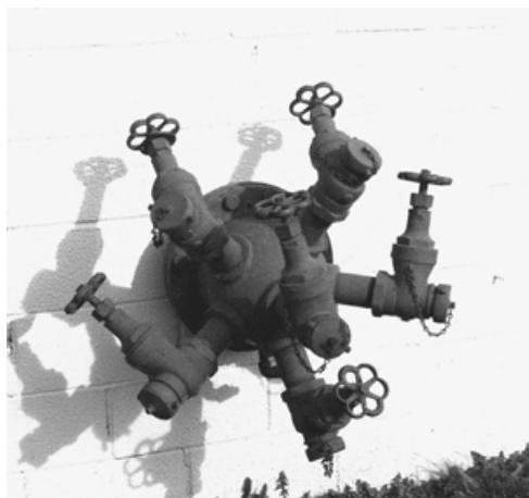
FIGURE 6.78 Fire pump test head.
