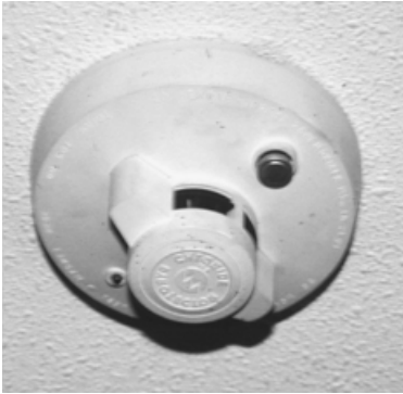
FIGURE 6.15 Combination smoke and heat detector.
