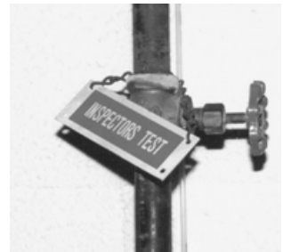
FIGURE 6.56 Inspector's test valve.
