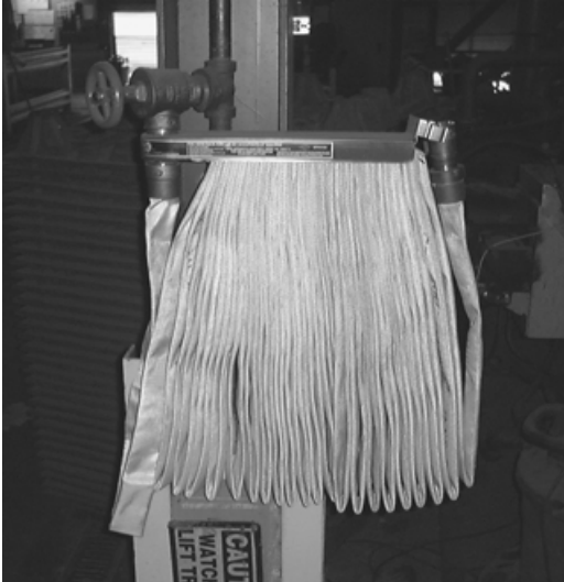
FIGURE 6.22 Hose station, rack.
