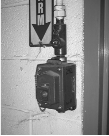
FIGURE 6.11 Pull station for hazardous location.
