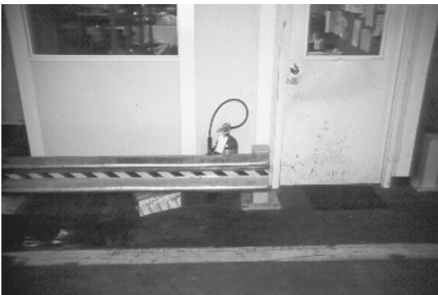
FIGURE 7.51 Extinguisher not properly mounted.
