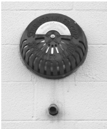
FIGURE 6.37 Water motor gong, outside building
