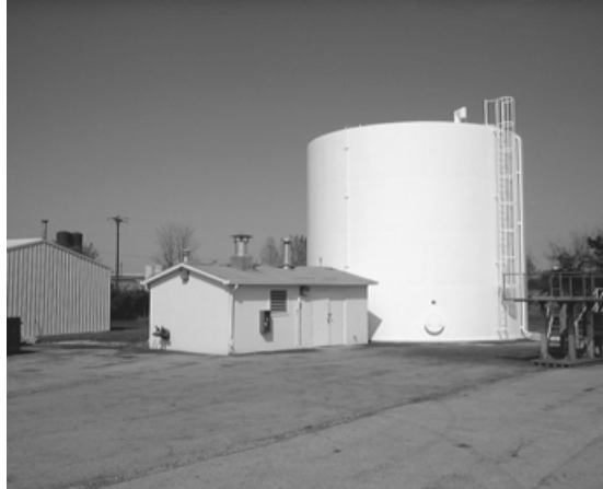
FIGURE 6.65 Suction tank and pump house.
