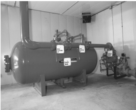
FIGURE 6.63 Foam storage tank. (Photo courtesy of Ansul Incorporated.)
