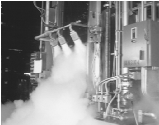
FIGURE 6.90 Carbon dioxide system discharge.
