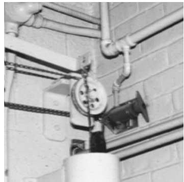
FIGURE 6.7 Fire door carbon dioxide system release.
