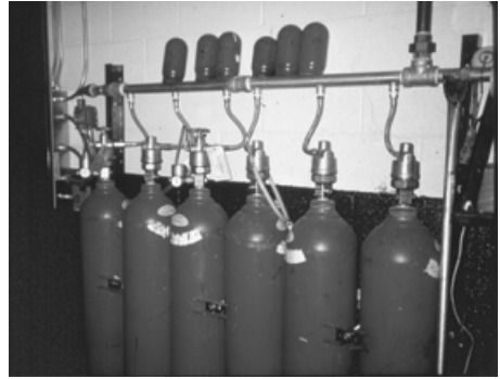
FIGURE 6.80 Carbon dioxide system high-pressure storage.
