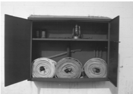
FIGURE 6.29 Hose house, wall mounted.
