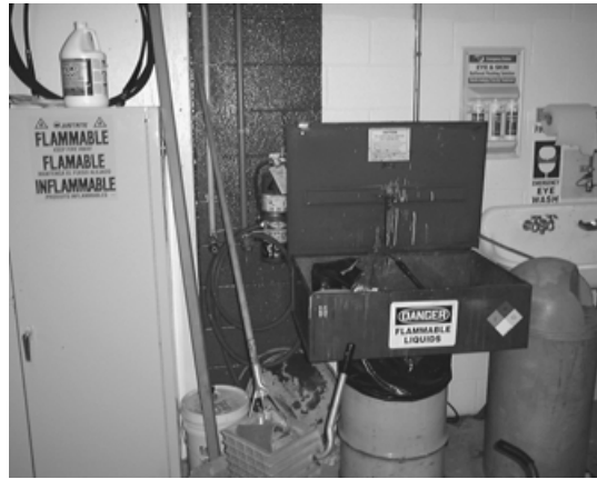
FIGURE 7.50 Obstructed access to extinguisher.
