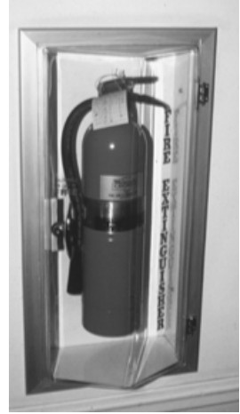
FIGURE 7.39 Extinguisher mounted in cabinet.
