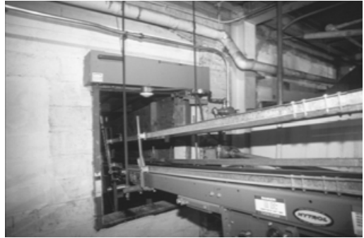
FIGURE 6.3 Fire door, conveyor pass-through.
