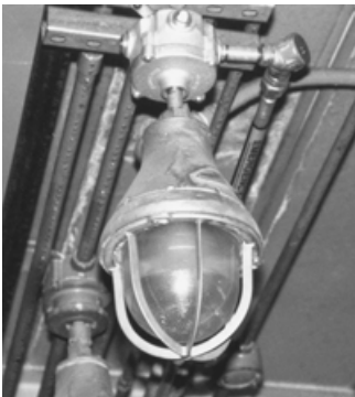
FIGURE 5.27 Explosion-proof light, incandescent.
